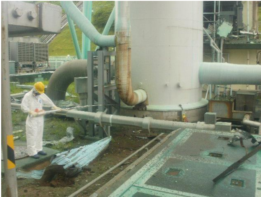
Location: Near the standby gas treatment system pipe joint at the bottom of the main exhaust stack of Units 1 and 2 Time: August 1, 2011, around 14:30 Photographed by: TEPCO
