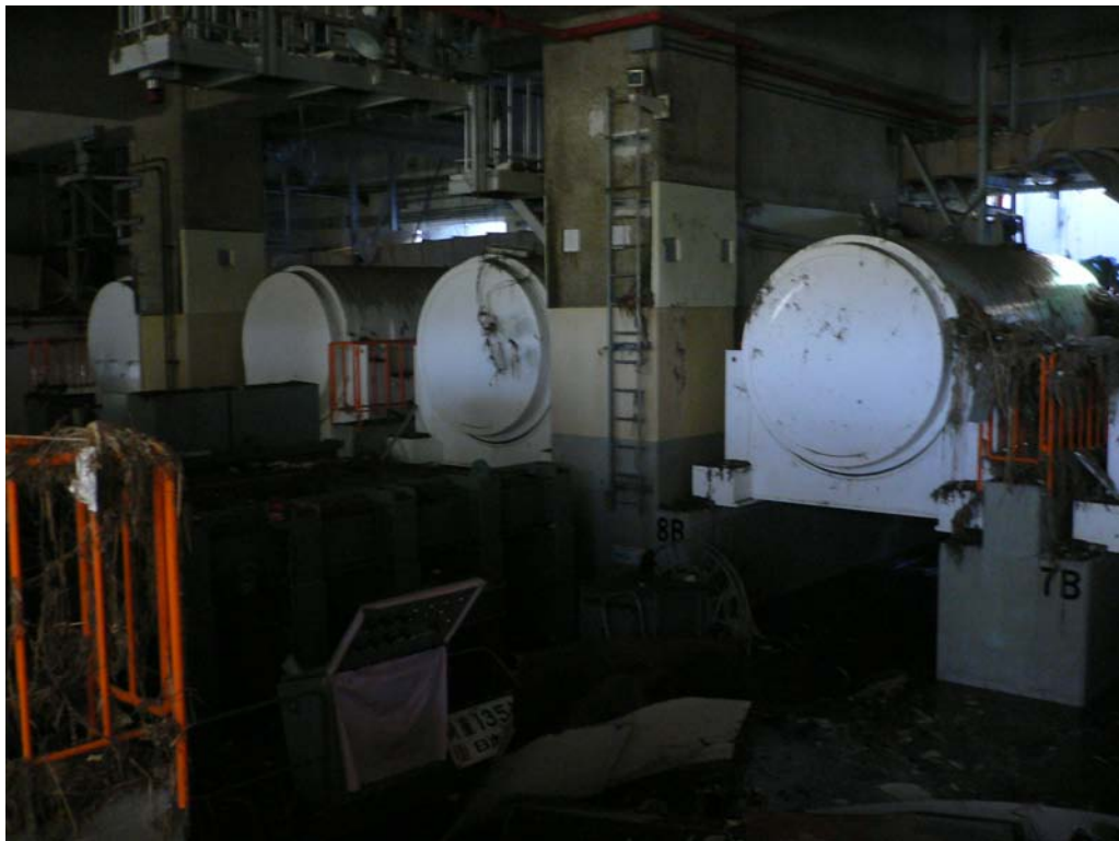
Figure II-2-56 Situation in Dry Storage Cask Facility
