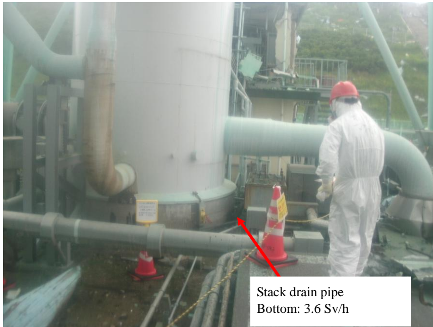
Location: Stack drain pipe at the main exhaust stack of Units 1 and 2 (view from the east side)
