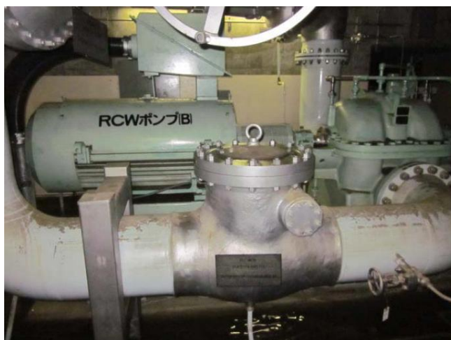
RCW pump (B) (after seawater was drained)
