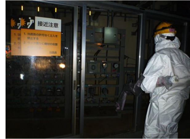
Reactor instrumentation rack
