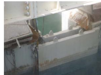
Spent fuel pool gate
