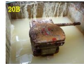
Fuel pool cooling and clean-up system valve
