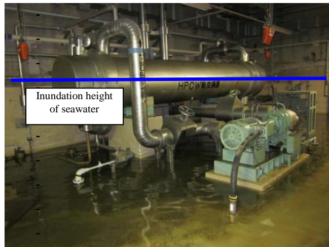
Seawater flooding in the HPCW heat exchanger chamber
