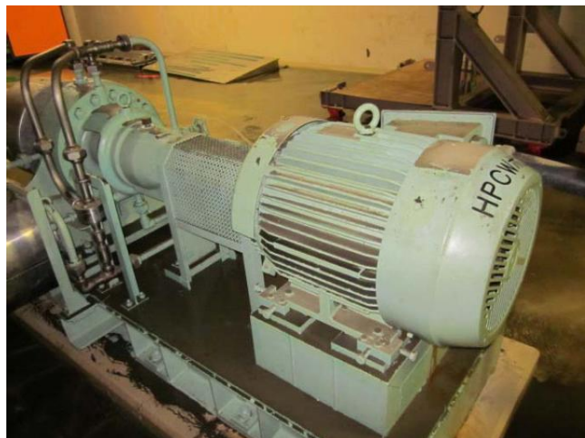
HPCW pump (after seawater was drained)
