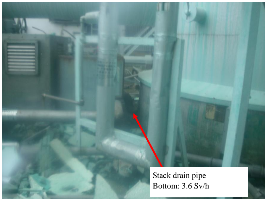
Location: Stack drain pipe at the main exhaust stack of Units 1 and 2 (view from the west side)
