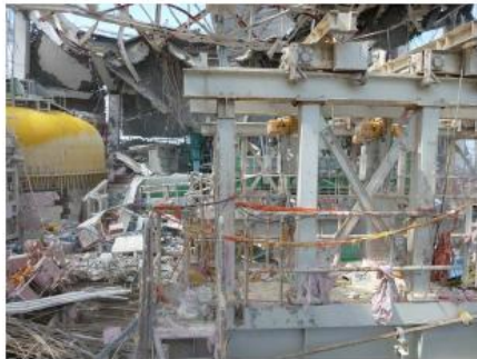
Equipment storage pool viewed from refueling carriage
